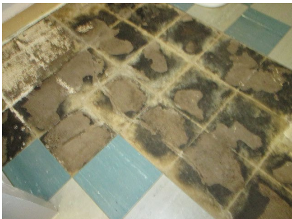
Figure 21 - Some of the mastic in Washroom 005 is exposed, including some loose. Loose material should be removed or sealed.
