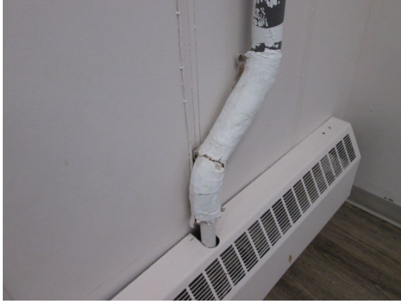
Figure 1 - Damaged pipe fittings in Room 001. Partially painted but some cracks, and some exposed parging adjacent wall.
