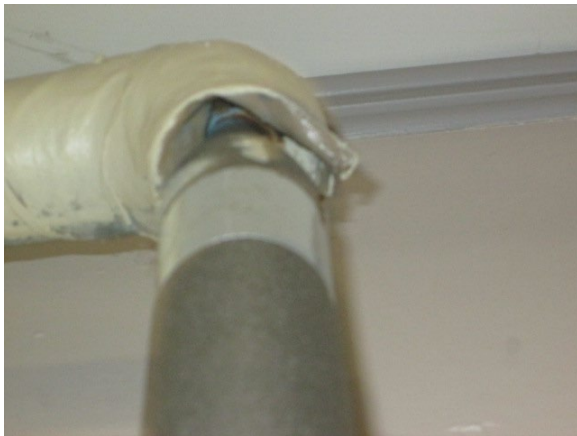
Figure 8 - Where the cover ends on two elbows in Room 005, some parging is exposed.
