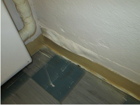
Figure 25 - In Basement Washroom 005 (shown) as well as Basement Hall 004, pale pink wall paint contains lead above the guideline. Some is also delaminating/flaking.
