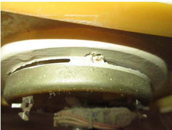
Figure 27 - The glass vial in the thermostat seen in Figure 26 has mercury present.
