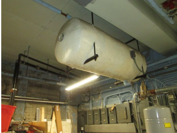
Figure 19 - The hot water tank in Boiler Room 010 also appears to have the same ACM insulation as the boiler.
