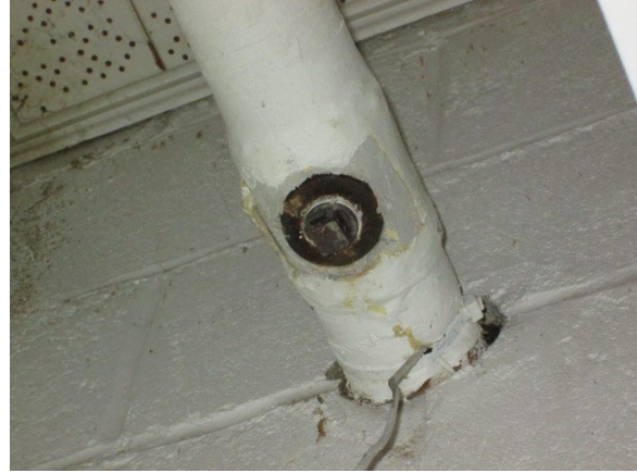
Figure 10 - The capped valve fitting in Room 007 has exposed parging that appears to be the same type as the asbestos-containing samples.
