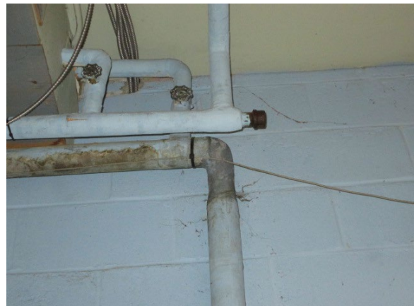
Figure 12 - Some fittings in Room 010 are slightly mouldy, and some minor cracking is adjacent these valve fittings.
