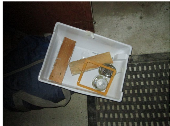
Figure 30 - The thermostat in Room 006 was found in a box as shown below.
