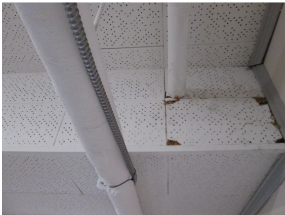
Figure 3 - View of pipes entering bulkhead in Room 001.
