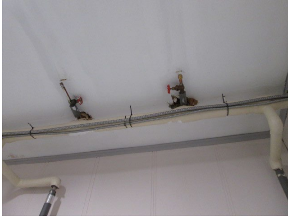
Figure 7 - Pipe insulation and fittings in Room 005. See the grey uninsulated pipe on either side in Figure 8 below.
