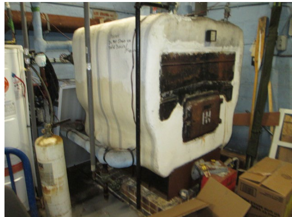
Figure 17 - The boiler in Room 010 is mostly in good condition. Also see Figure 18.
