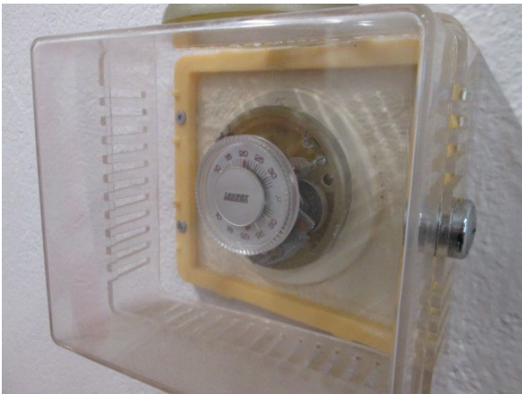
Figure 26 - The Lennox thermostat in Room 001 near Hall 004 has a mercury vial switch. See Figure 27.
