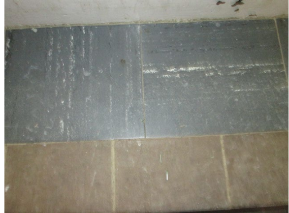
Figure 22 - 9"x9" dark grey floor tiles on the stairs in Stairway 006A contains asbestos per Sample 10.
