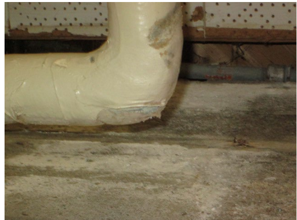
Figure 5 - Some of the covering on the pipe elbow in the back right of Room 003 is incomplete, and should be re-covered or otherwise sealed.
