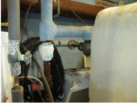
Figure 13 - Location of partially repaired pipe fitting in Room 010. See Figure 14 below.
