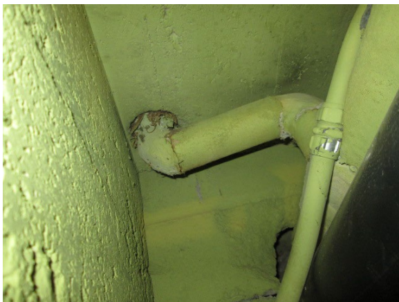
Figure 15 - Fittings to left side of doorway to Room 011 (storage under stairs). The elbow to the left is partially painted but has some exposed parging, and the elbow to the right is cracked at both ends.
