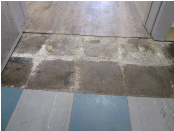
Figure 20 - Both 9"x9" floor tiles in Washroom 005 contain asbestos, as does the mastic underneath. Similar conditions were observed at the doorway of Room 007. Also of note, the wood click laminate in the hall and elsewhere may cover older floorings such as shown.
