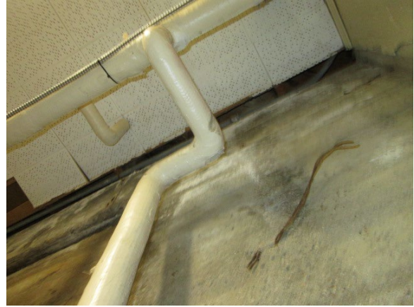
Figure 4 - Pipe elbows in Room 003.
