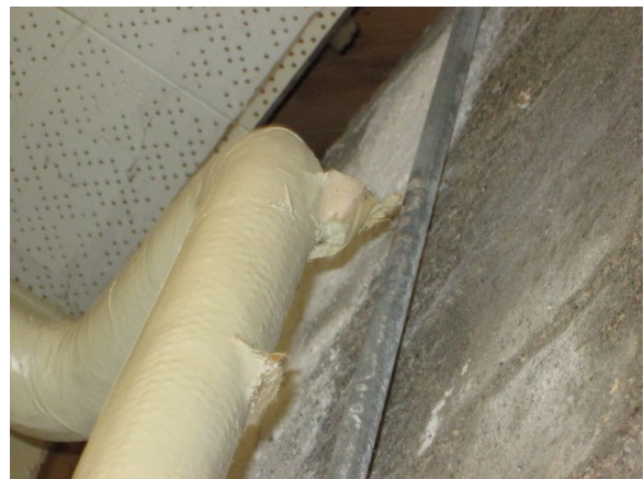
Figure 6 - Some of the covering on this pipe elbow in the back left of Room 003 is damaged.
