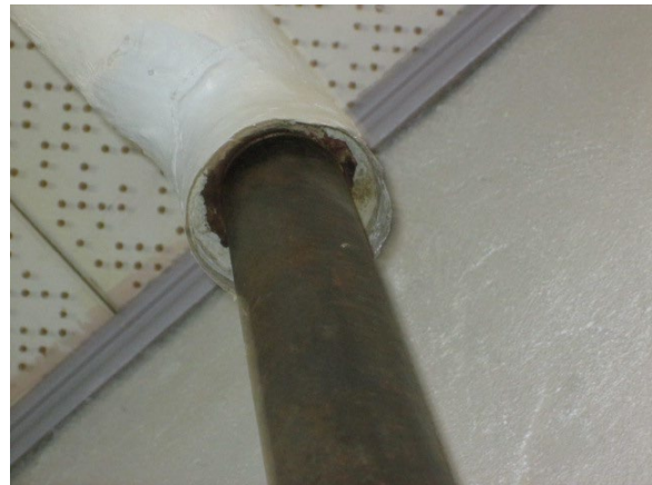
Figure 11 - Pipe elbows in Room 008 (shown) and 009 have exposed parging due to incomplete coverings.
