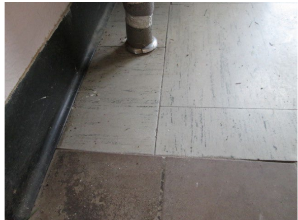
Figure 23 - 12"x12" light green-beige floor tiles on the landing of Stairway 006A also contain asbestos in the tile and mastic. See Sample 11.
