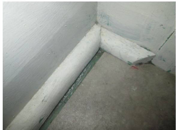
Figure 24 - A sliver of green floor tile was observed underneath stick-on vinyl sheet flooring tiles in Room 105A. Sample 12 shows that these tiles also contain asbestos, and therefore could be underneath other visible flooring.
